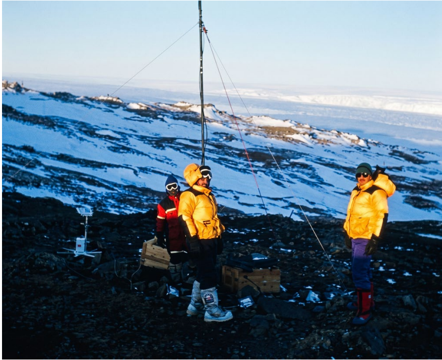
Installation of Repeater station for HF communication in Vetaiha peak
