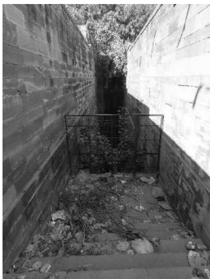
Anwana Baodi-going down the dirty stepped corridor
