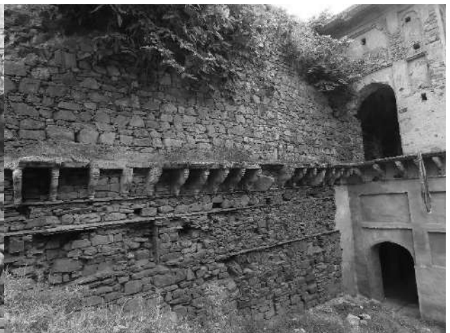
Manoharpur Baodi-ledges supported on brackets on the side wall in bad condition
