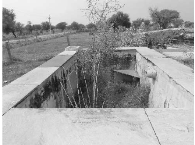
Lakshmangarh-Dholas ka Kua-water tank with gaumukh outlet
