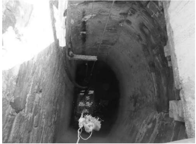
Merta City-Suwa Baodi-auxiliary well behind the main well shaft
